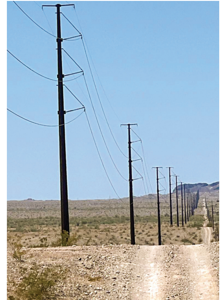
Example of 230-kV Transmission Line, as described.
