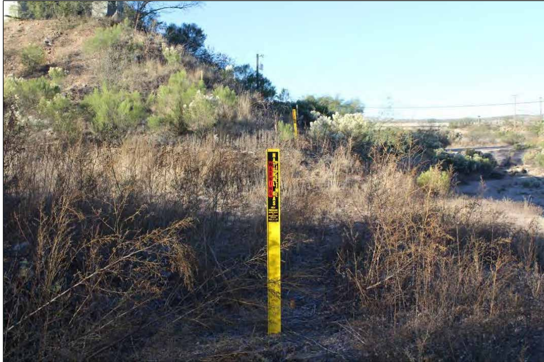
Natural gas pipeline on the southeastern side of Mariposa Canyon Wash in section 5
