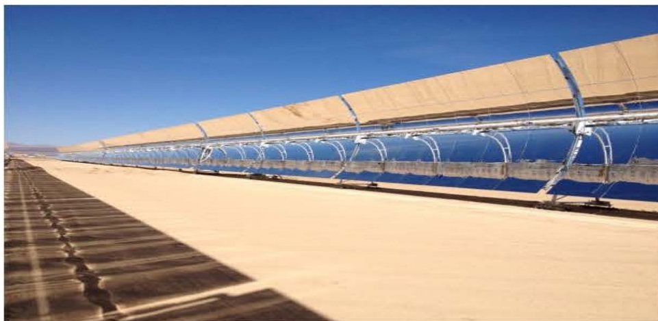
Mohave Solar Collectors
