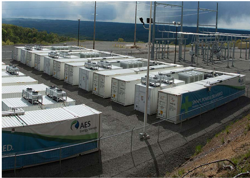
AES Storage LLC's Laurel Mountain Energy Storage Supplies 32 MW of regulation using Li-ion batteries
