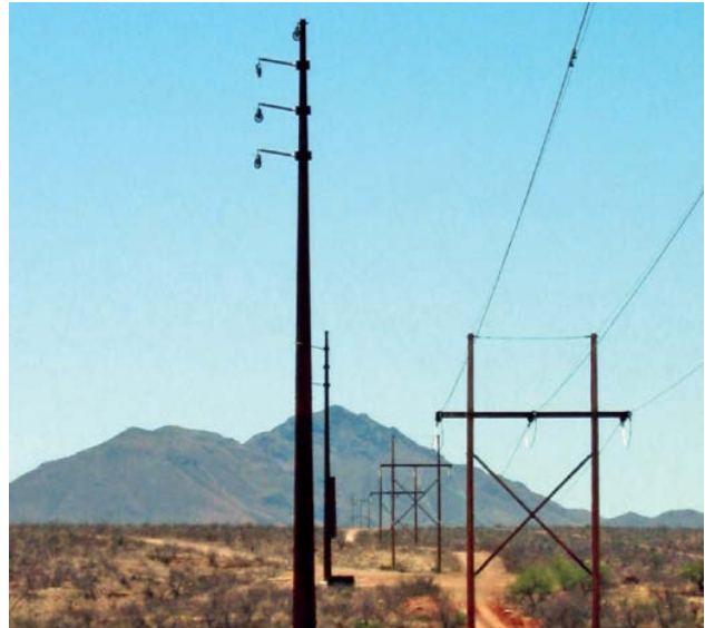
Comparison of the recently installed steel monopole structures alongside old wooden "H-frame" structures along the Vail to Valencia Transmission route. The H-frame structures will be removed after construction of the new facilities in 2014.
