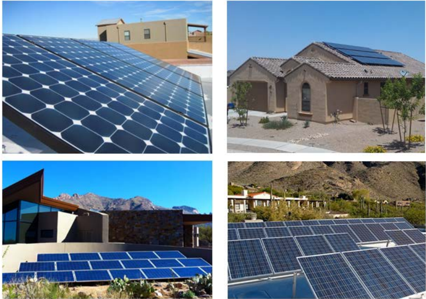
Typical residential distributed photovoltaic (PV) systems
