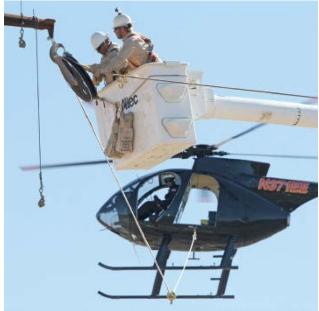
UNSE journeymen Nic Lyons and George Molina and helicopter pilot Jeffery Wojtowicz prepare to pull the new 138kV transmission line on the Vail Valencia Project
