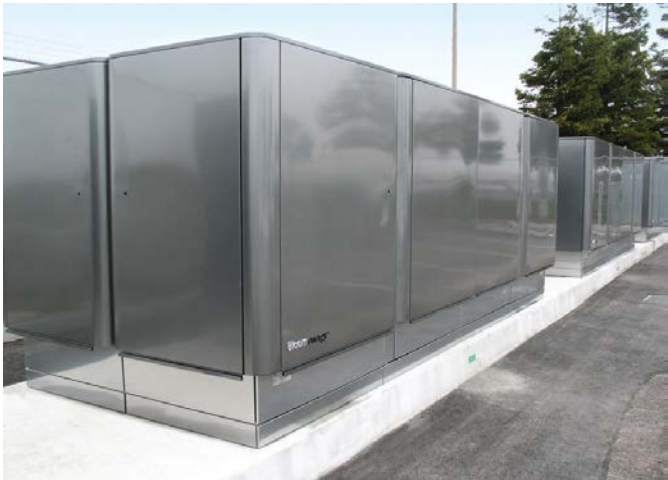
Typical Installation of Bloom Box Units Source: Bloom Energy
